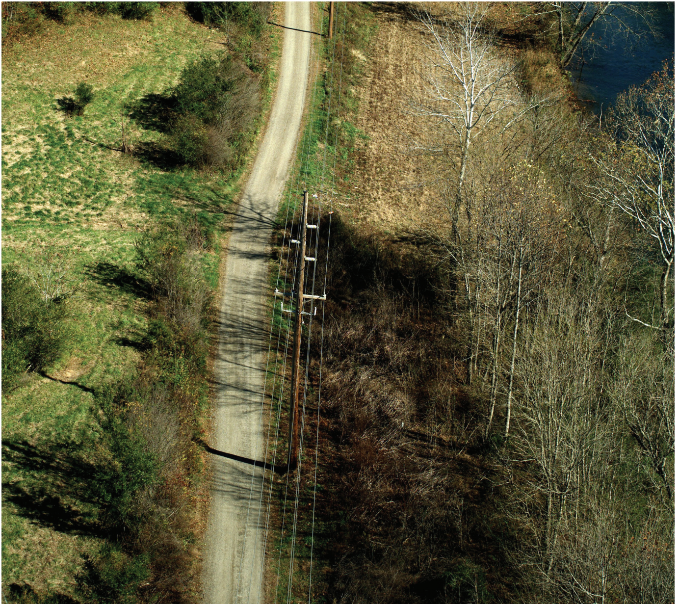
Existing Fieldale - West Bassett No. 1 69-kV Line Monopole with Post Insulators and Cross Arms
