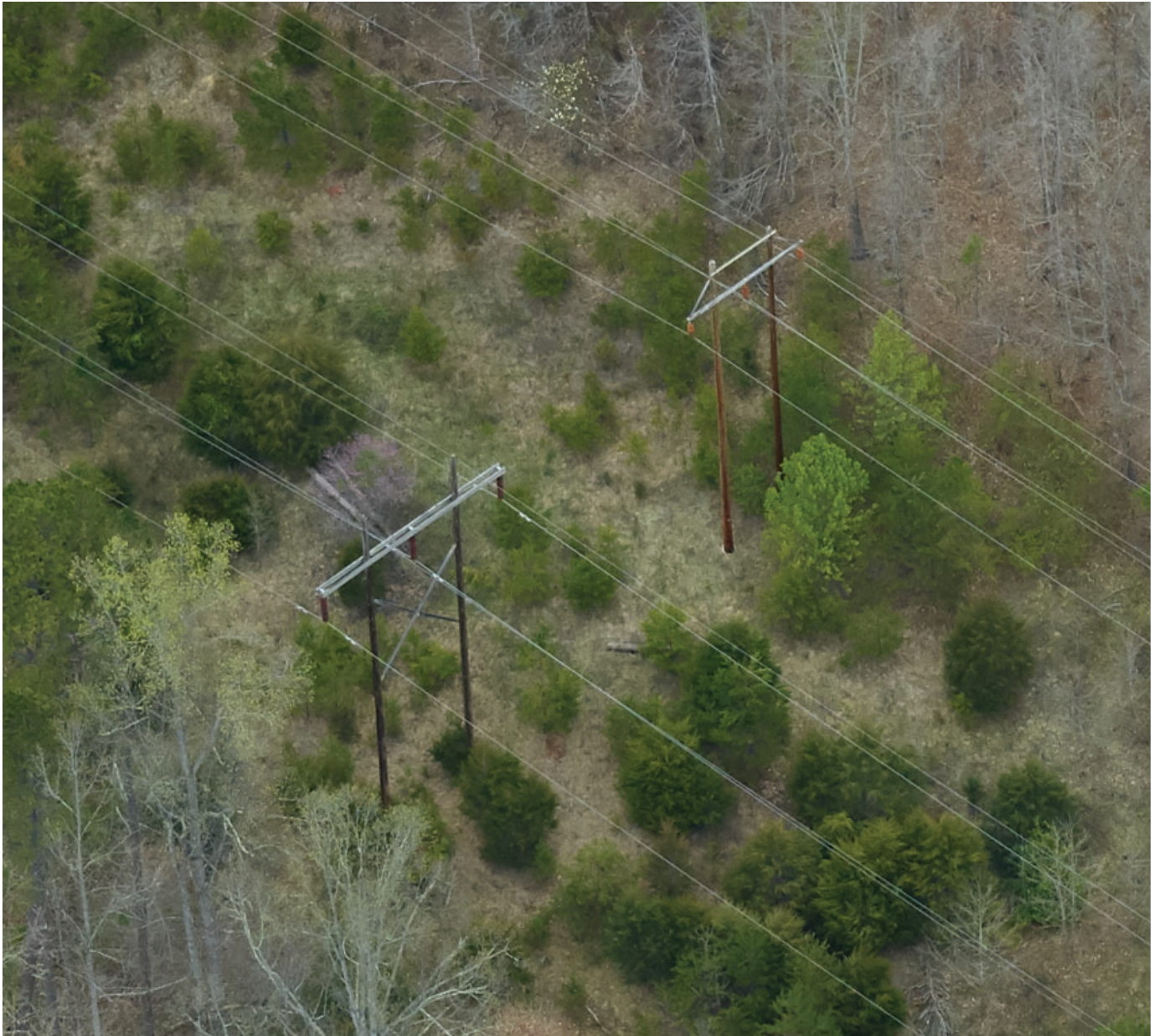
Existing Claytor - Fieldale 138-kV Line (Left) and Fieldale - West Bassett No. 2 69-kV Line (Right) H-Frames
